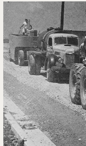
Laying the base course on a street of a Capehart Housing project at the Richards-Gebaur Air Force Base at Grandview, Missouri. A Cat 12 motor grader is followed by a watering truck and a Ferguson 25-ton roller.
